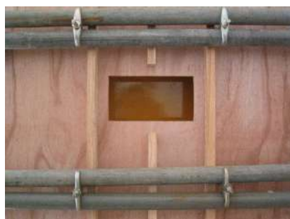
(1) Hole in sheathing board
