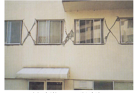
(c) 短柱のせん断破壊
